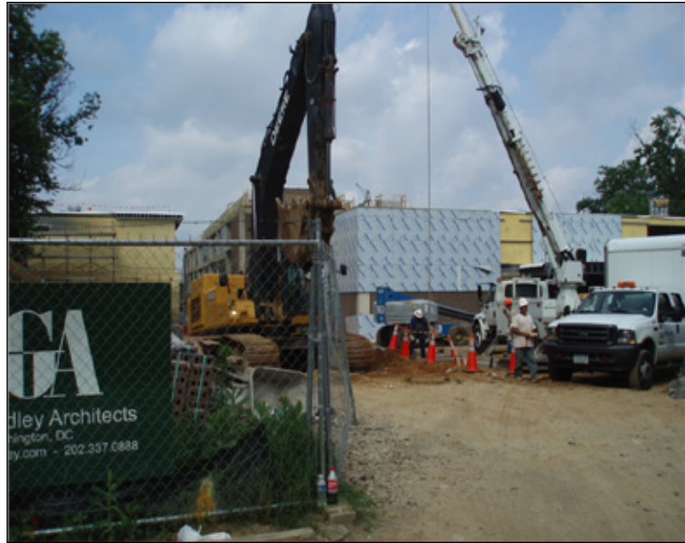
Addition on a 1960s public school, being modernized in 2009 (Source: 21st Century School Fund, 2009).
